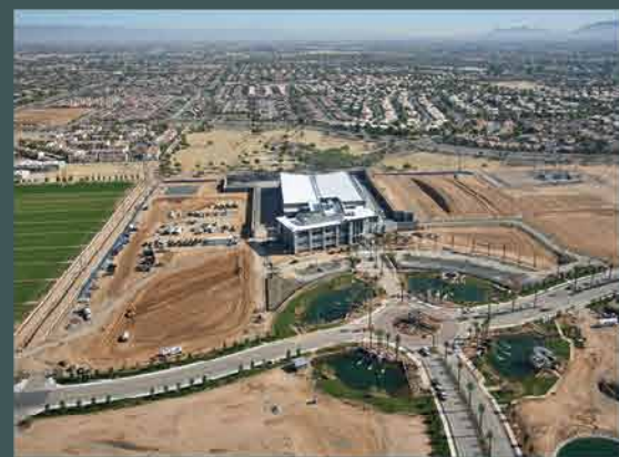
CyrusOne selected general contractor JE Dunn Construction Company to oversee building its 186,500-sf data center—which would normally be accomplished during an 18-20 month timeframe—in a record seven months.
