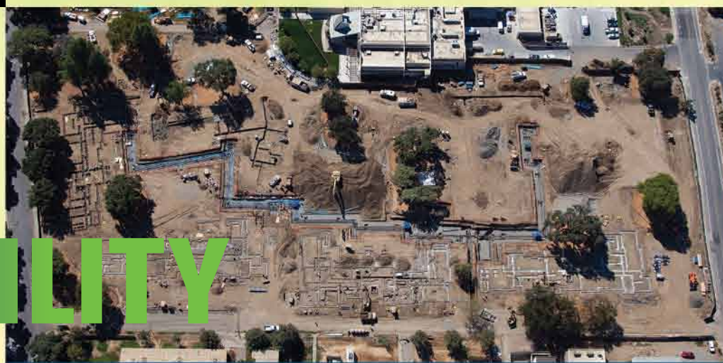
Bergelectric has helped to accelerate this $75-million UC Davis Tercero Student Housing Phase 3 project through an intensive design-review process and phasing electrical construction.
